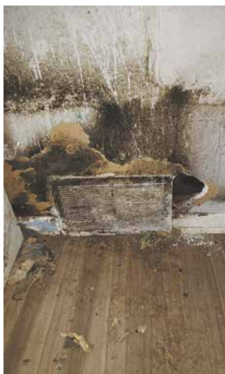
Wall behind the fridge with a rathole in it.
