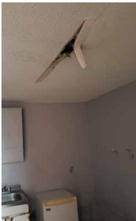
Hole in the ceiling where the water leaked.
